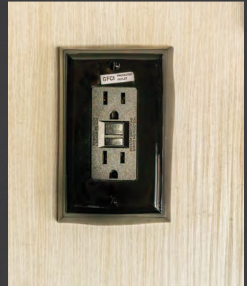
GFI Protective Outlet
