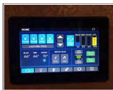
Figure 5-7: Water heater screen (Spyder control system)
