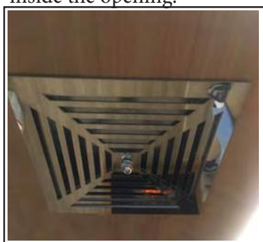
Figure 3-2: Outgoing air vent
