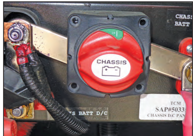
Figure 9-16: Engine battery disconnect switch
