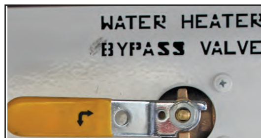
Figure 13-9: Water heater bypass valve
