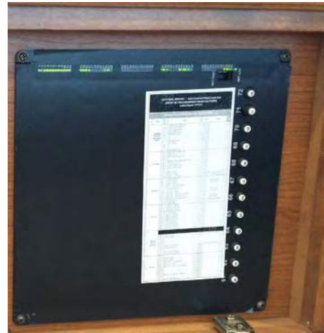
Figure 9-3: Multiplex System Switch panel
