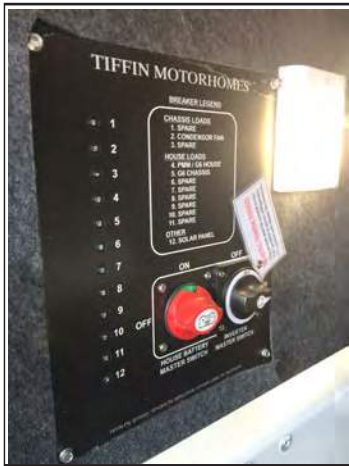
Figure 9-15: House battery disconnect switch
