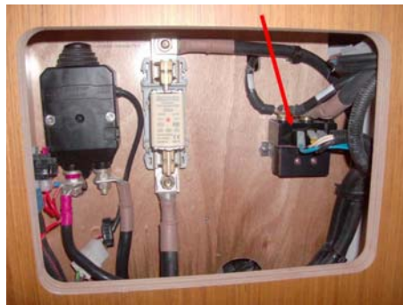
Operation relay Under the bed - Forward cabin
