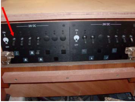
Breaker 120A Location: Starboard saloon
