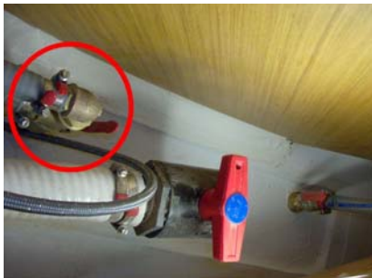
Shower + Washbasin Port aft head compartment
