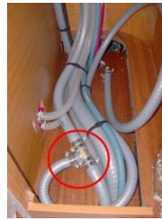
Drainage - Dishwasher: Connector to sink drain in kitchen cabinet.
