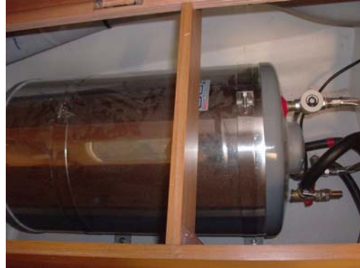
220V 60L WATER HEATER Location: Saloon - Starboard
