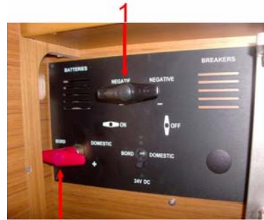
Battery switch 24V Location: Saloon 1. - Common 2. + Service
