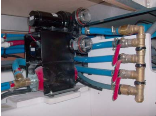
WATER PUMP 24V Location: Saloon - Central
