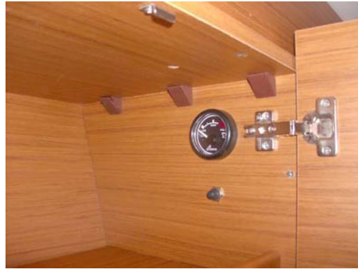
Excrement tank gauge + Control - Drain to sea Location: Cupboard - Head version
