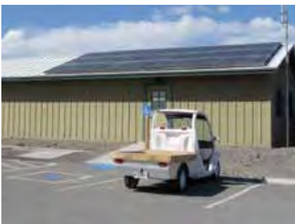
SunWize 6kW Grid-Tie System #999GTS670 INSTALLED BY: National Park Service
