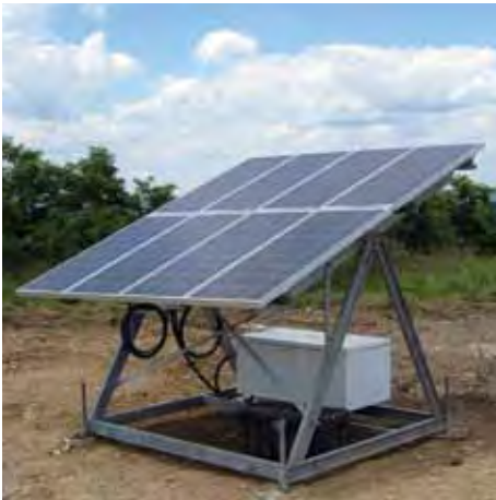
SunWize 880W Power Station
