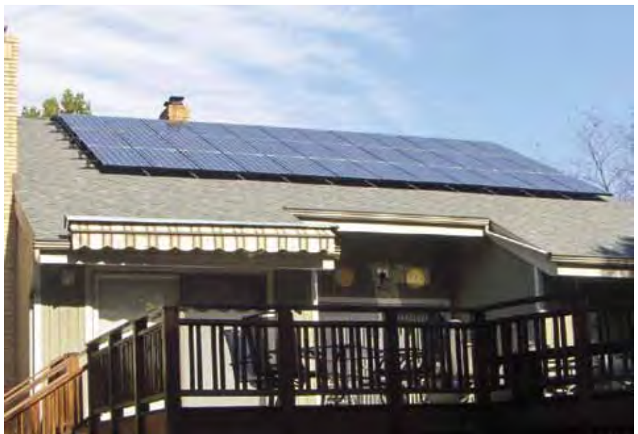
SunWize 7.7kW Grid-Tie System #999GTS1965 INSTALLED BY: Dan Hicks, Sun Saver Solar Systems
