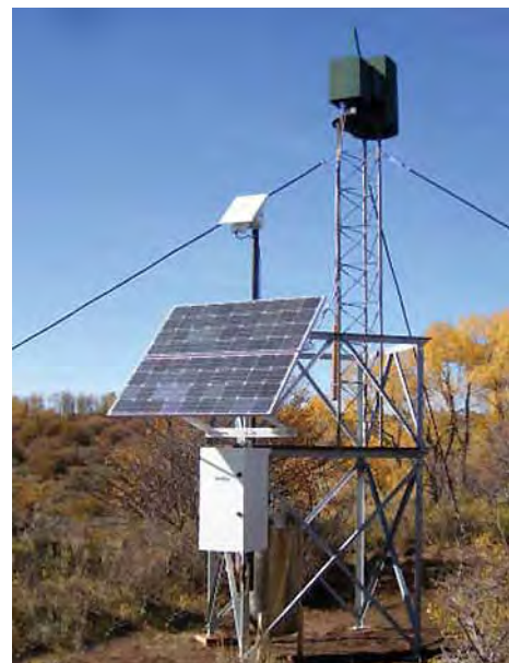
This SunWize Power Ready PR230, located in central Wyoming, powers weather modification equipment (cloud seeding)
