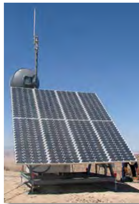
This 1200 watt SunWize Power Station located in a remote location, powers telemetry equipment
