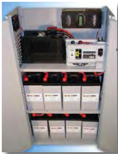
All components are housed in a lockable, vented, indoor enclosure with thermally active cooling fan (shown with top removed for display)
