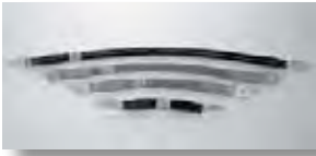
SW Battery Cables
