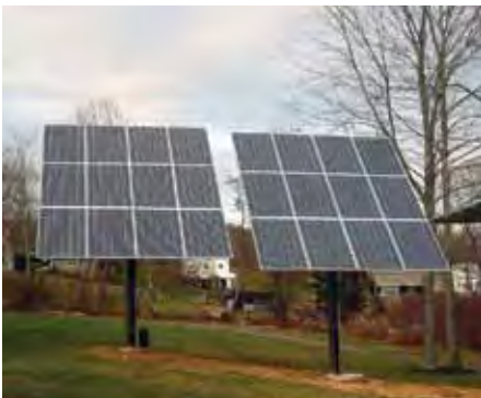
SunWize Grid-Tie System #999GTS440-Z no rack INSTALLED BY: Giuffrida Electric Company
