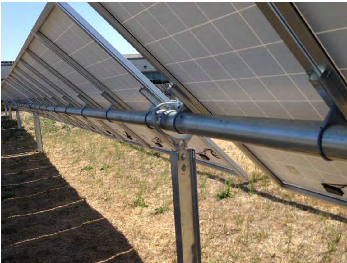
Photo 7. The back of the solar panels.
