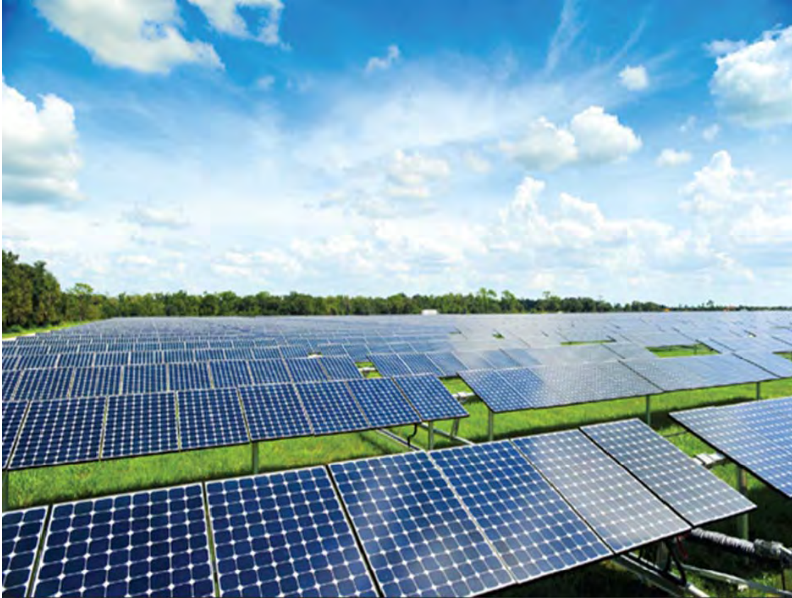
Photo 6. Single-axis, tracking photovoltaic system with panels close to maximum tilt as viewed from the east or west.
