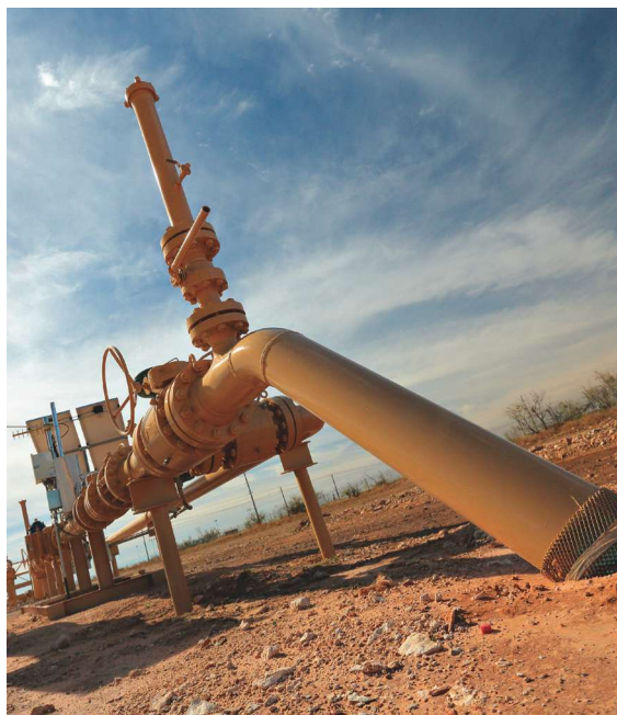
Multiple valves make up a meter run connecting a Permian Basin well pad to a gathering system. (Photo courtesy of Navitas Midstream Partners LLC)
