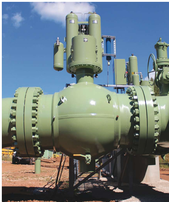
The bustling Marcellus Shale has emerged as a major valve market as the midstream plumbs Appalachia, linking what may emerge as the world's largest gas field with major North American markets. (Photo courtesy of MRC Global Inc.)
