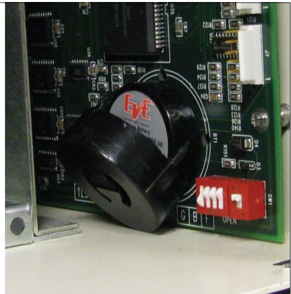
B. Battery Cover Dislodged
