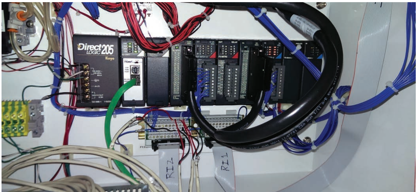
Figure 2: The new AutomationDirect Do-more PLC worked with all the existing I/O modules and wiring.
