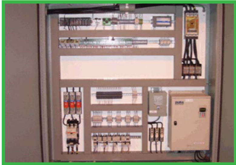
Figure 1, Steel Processing Machine Control Panel
