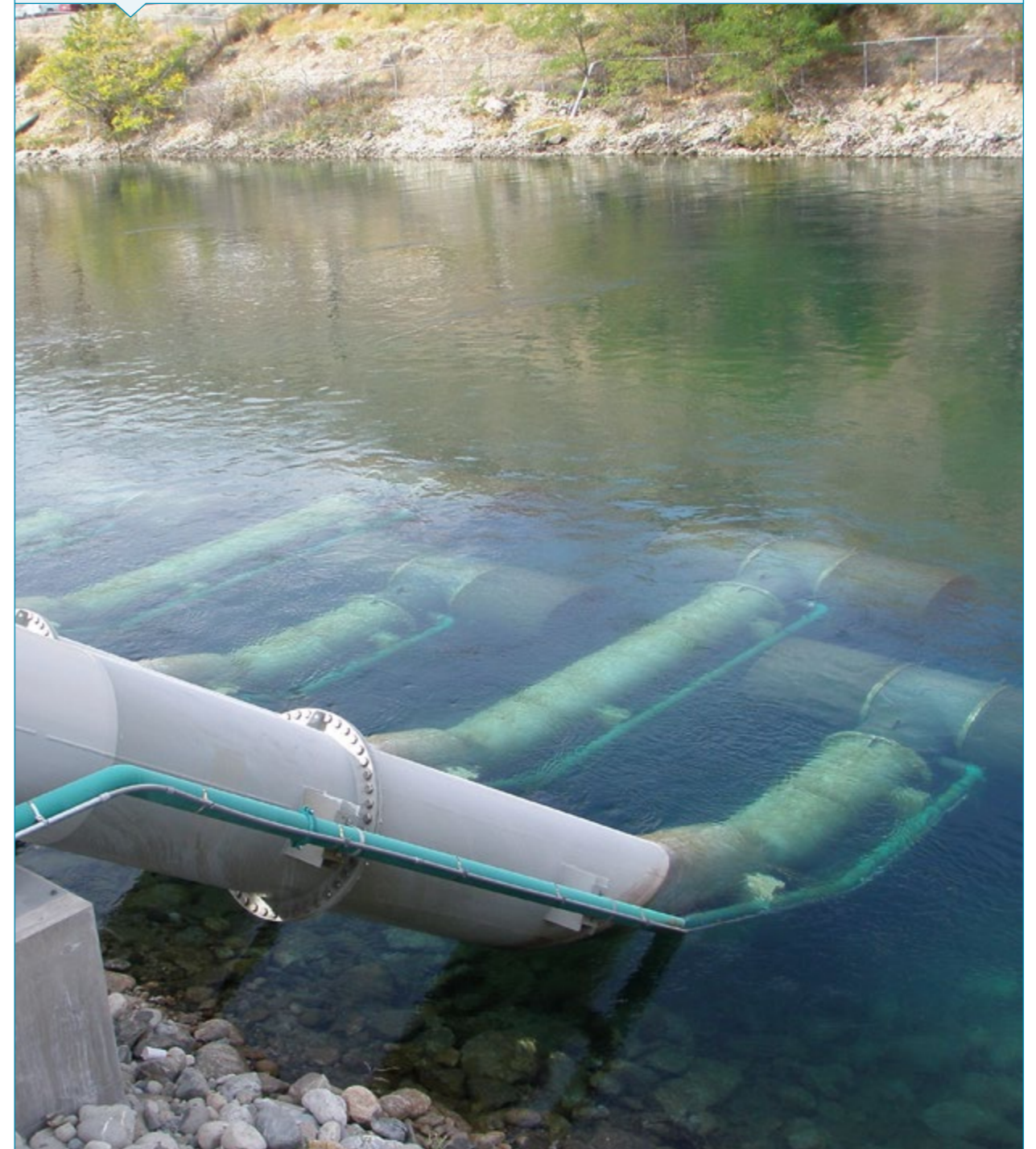
Irrigation with Flygt axial flow pumps
