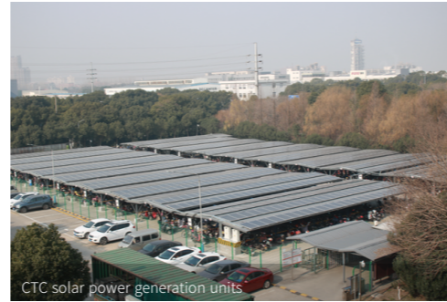
CTC solar power generation units
