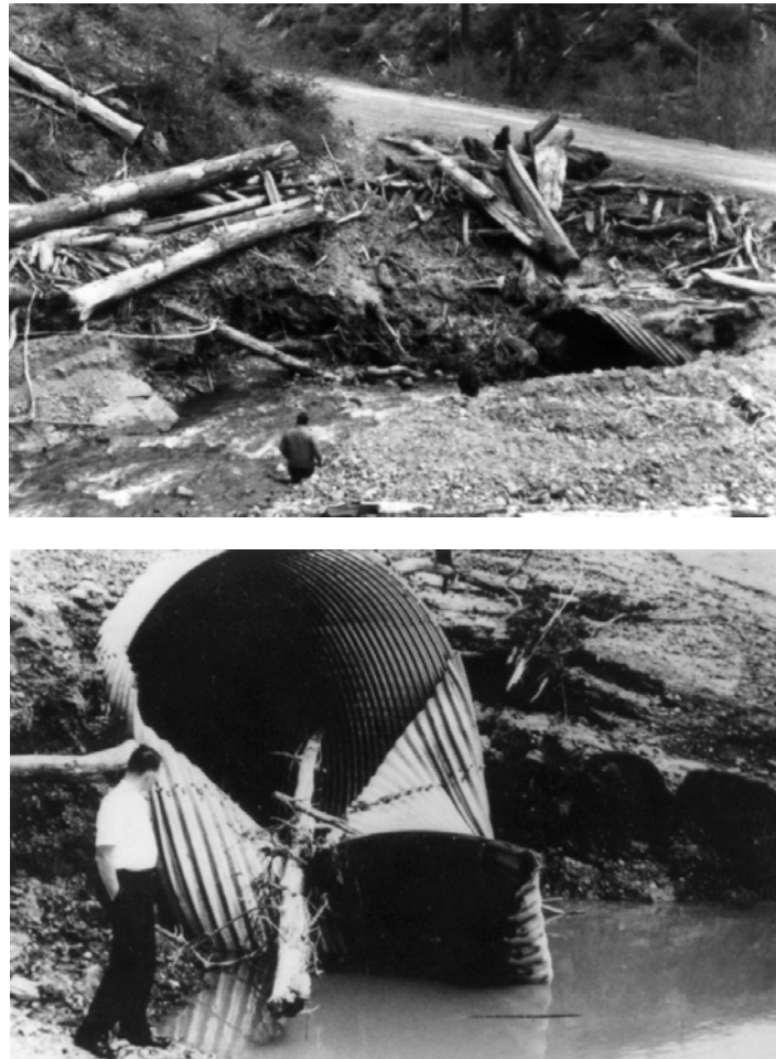
Figure 9.17 Damage to Culvert Inlets Due to Hydraulic Forces and Drift
