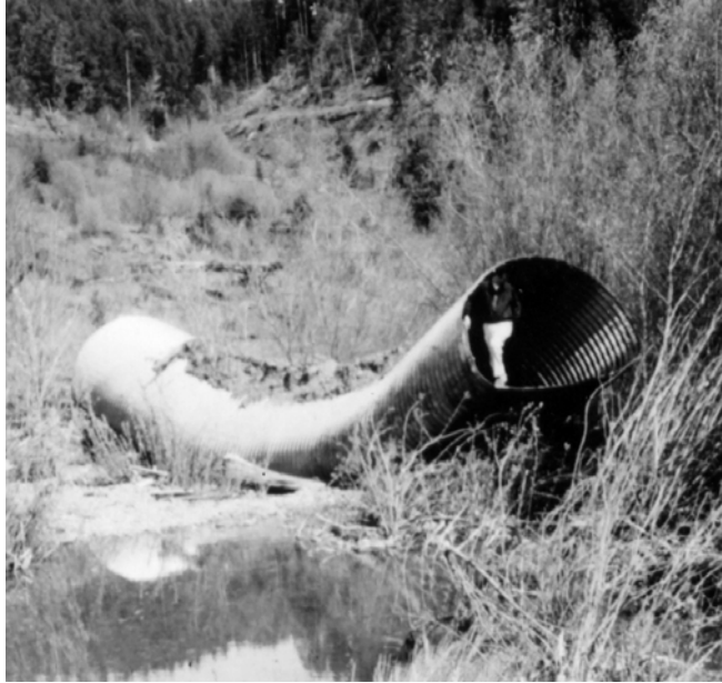
Figure 9.18 Culvert and Roadway Fill Failure from Buoyant Forces: Culvert Carried Downstream
