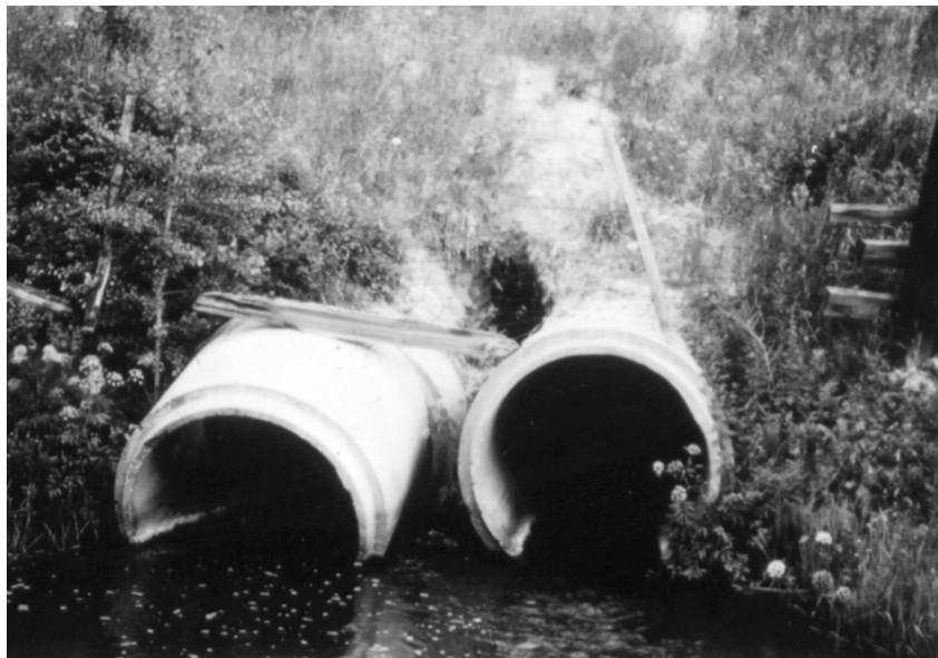
Figure 9.19 Void From Piping Along Culvert Barrel
