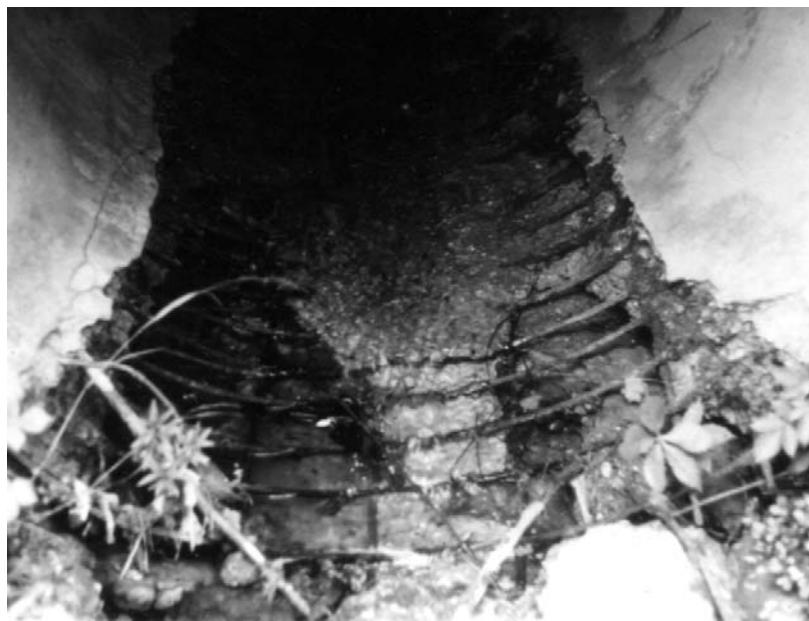
Figure 9.25 Loss of Culvert Material from Abrasion
