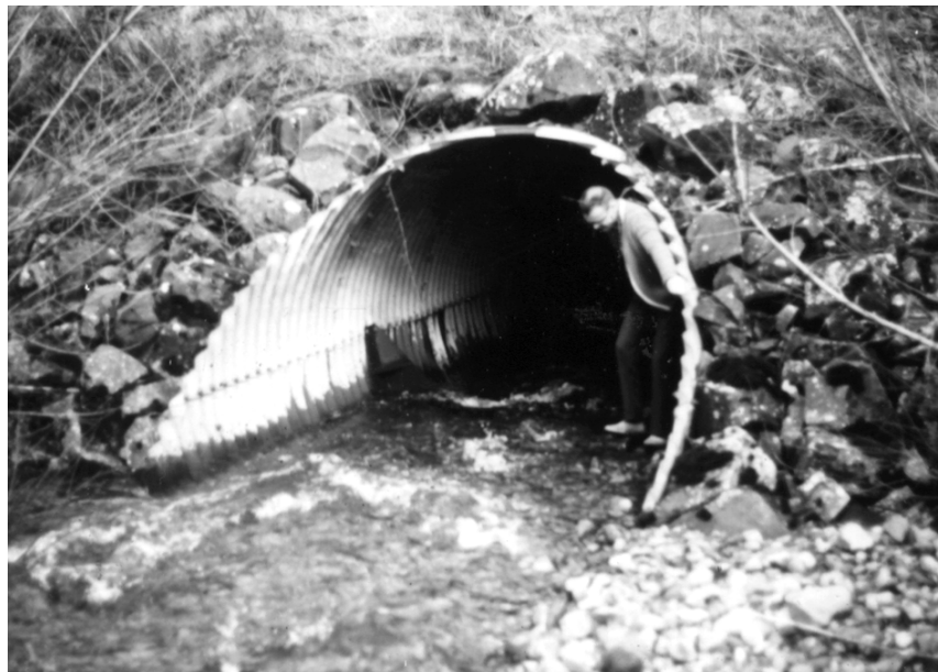
Figure 9.23 Culvert Invert Placed Below Streambed Baffles used to hold gravel in place and provide natural stream bed for fish passage
