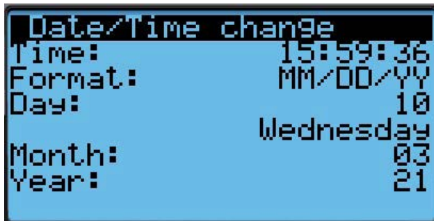
FIGURE 35 Setting Controller Date and Time
