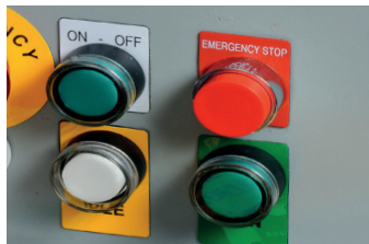
Control panel labels
