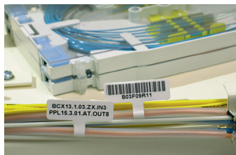
Fibre optic cable markers
