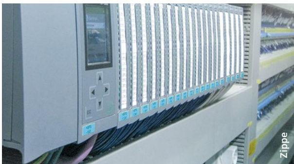
Simatic S7-1500 Advanced Controllers from Siemens have become established as the foundation of more complex automation solutions for Zippe batch plants.
