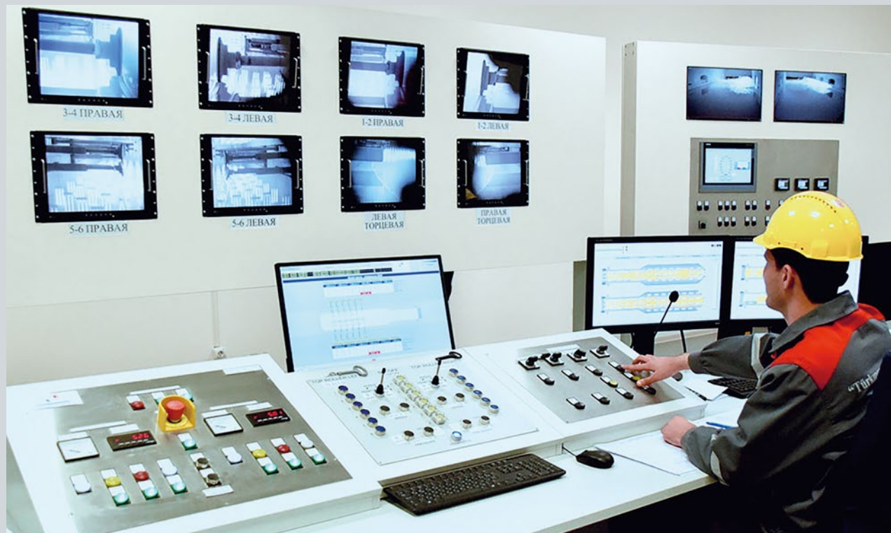
Operators value the plant-wide integrated automation based on the Simatic PCS 7 process control system.
