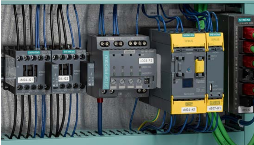
Figure 6-61 Example: Reference designations on various items of equipment in the control panel
