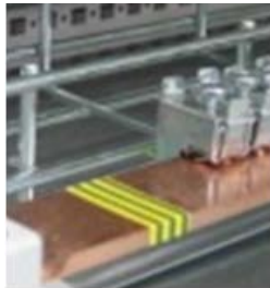
Figure 6-50 Example: Bicolor combination GREEN-AND-YELLOW at the end of the grounding bar
