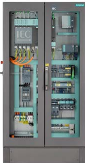
Figure 6-18 Control panel with appropriate enclosure
