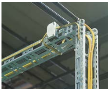
Figure 6-24 Cable freely installed on cable rack
