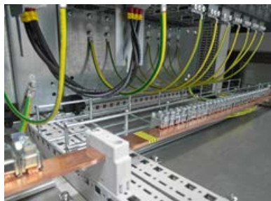
Figure 6-68 Example: Marking with GREEN-AND-YELLOW at the end of the protective conductor busbar
