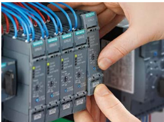
Figure 7-10 SIRIUS 3RM1 motor starters in the control panel
