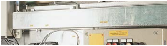
Figure 6-25 Cable installed in cable duct
