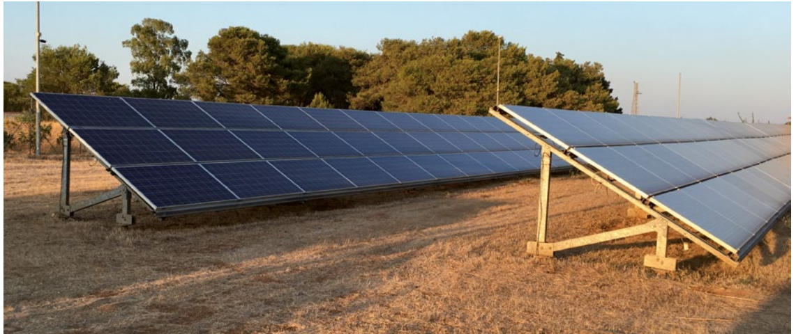
Figure 90 panel of PV module in landscape conditions
