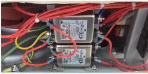
Two EMC filters fitted, Heater & Microwave*
