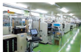
② "Highly reliable SMT" line
