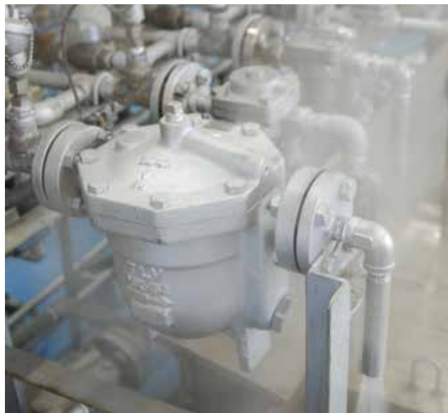
▲ Figure 2. Before starting the steam-trap management program, the plant should evaluate the current steam-trap practices and determine whether the optimal technologies are being used.
