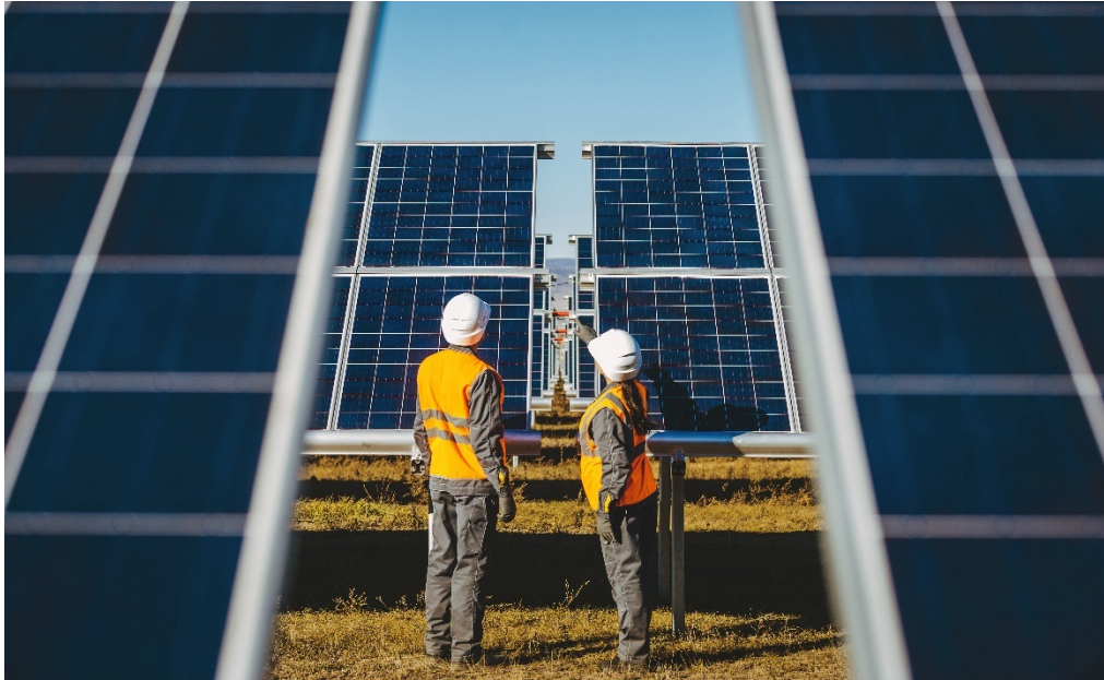
Figure 3-12: Representative Photo of Single-Axis Tracking PV System in the Morning, Facing East
