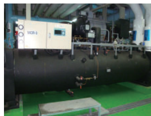
High-efficiency chiller installed by Sony Electronics (Wuxi) Co., Ltd. in China
