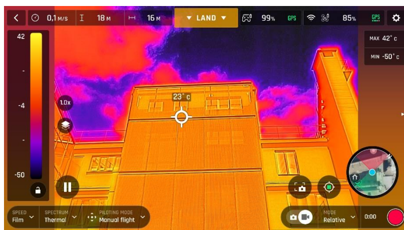
Temperature scale has not been locked from reference image; the scale has adapted to the new scene (- 50 to 42° C), the colors of the building now lack contrast, but the clouds and sky have been colored.
