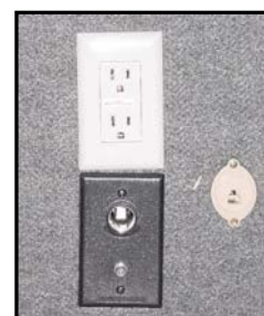
Figure 7-6. Typical 12VDC Receptacle (Bottom)
