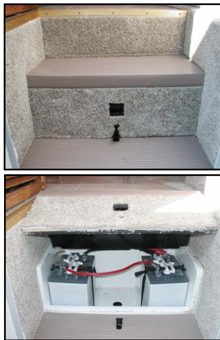
Figure 7-3. Stairwell (Top) and Battery Storage Underneath (Bottom)
