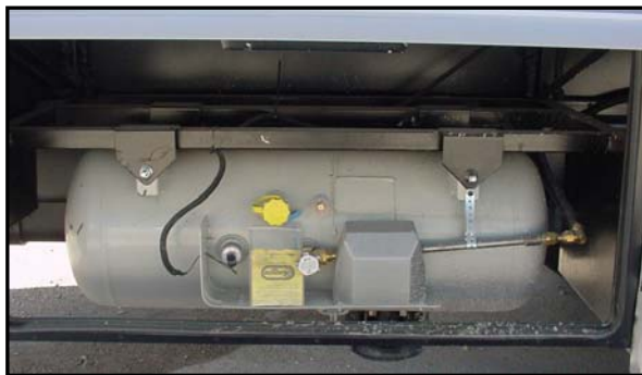
Figure 2-4. Liquid Propane Tank
