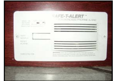
Figure 3-5. CO/LP Gas Detector
