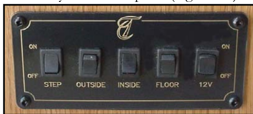
Figure 7-4. Battery Disconnect Panel
