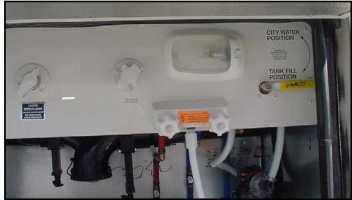
Figure 11-6. City Water Connection
