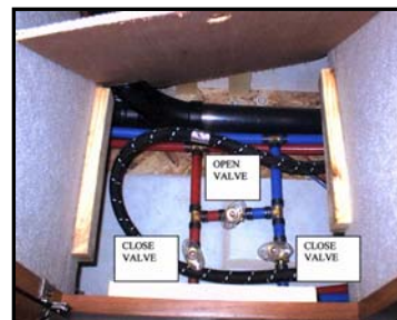
Figure 4-14. Water Heater Drain
