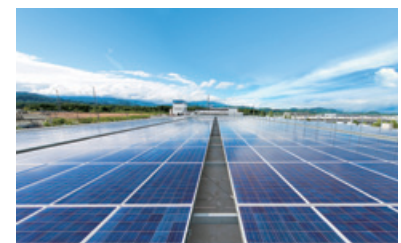
Solar Power Generating facility of Koriyama Second Office
