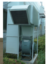
Exhaust vent with a noise reduction cover
