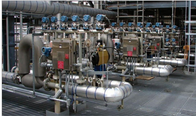
Figure 11: Hydrogen / natural gas blending system.
