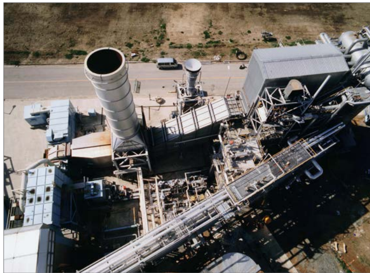
Figure 13: High hydrogen fueled 6B.03 gas turbine.
