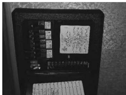
Figure 9-1: Circuit Breaker Box
