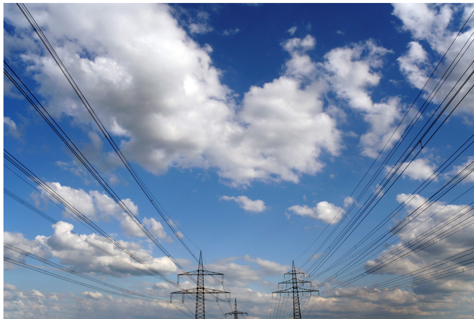
Figure 1. AC transmission lines.
