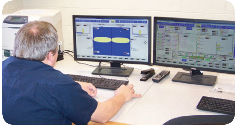
The new system leverages the Rockwell Automation® PlantPAx Process Automation System – an integrated control and information solution.
