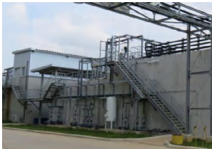
Industrial water and wastewater treatment plant (Indonesia)
