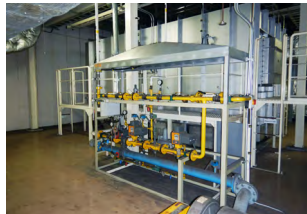
Deodorizing equipment for electrodeposition drying furnaces to reduce VOC emissions (Okazaki Plant)
