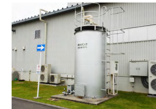
Rainwater storage tanks (Okazaki Plant)
