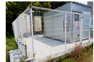
Groundwater membrane filtration equipment (Okazaki Plant)
