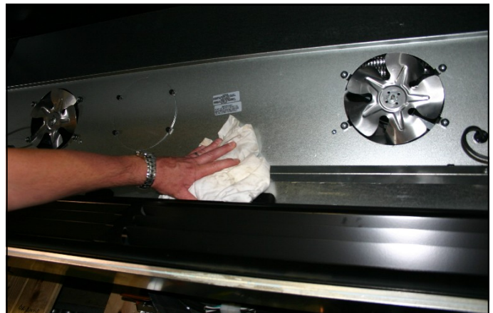
Image #7 Clean under Air Return Grille and Fan Shroud Area with moist cloth. Remove drain cleaning access door and clean drain.
