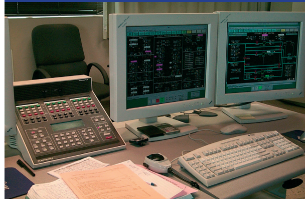
Dual CRT flat panel Ovation® Operator workstations are used to efficiently monitor and control the Sacramento Regional Wastewater Treatment plant processes.
