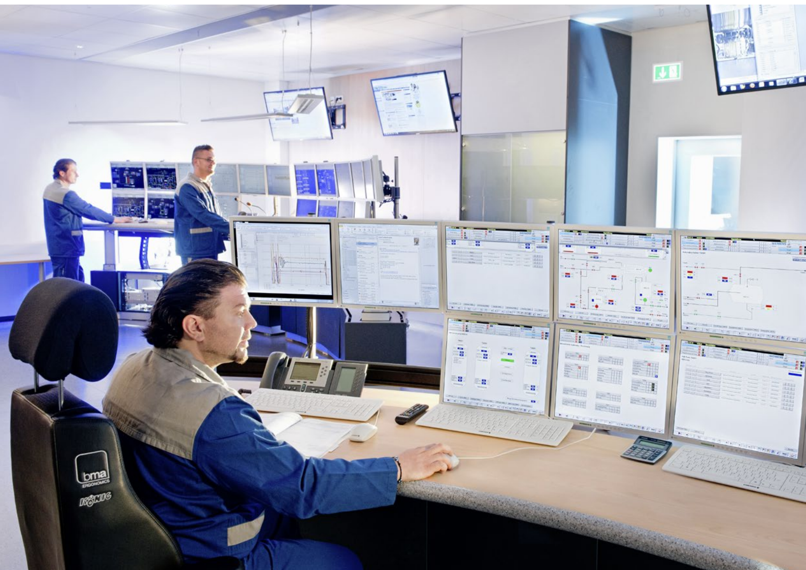
The production plants are monitored from the control center
