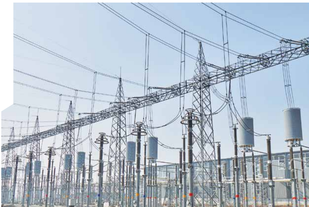
400kV Air Insulated Substation at Rajasthan
