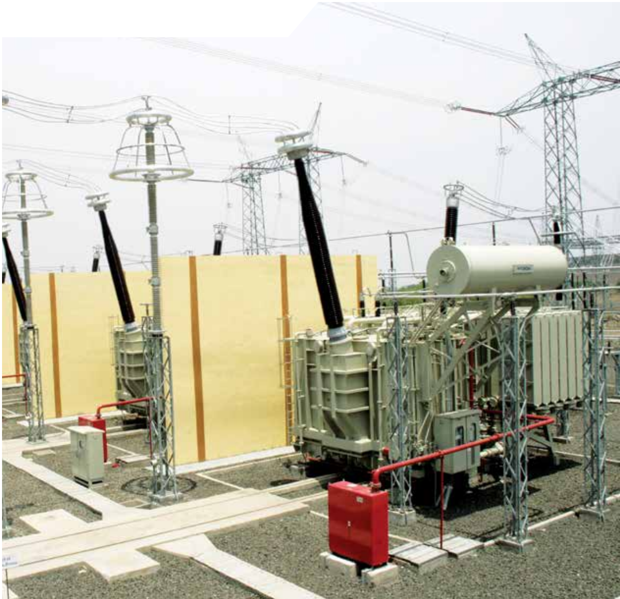
500 MVA, 765/400kV, 1 Phase ICT with fire fighting system for Sterlite Grid
