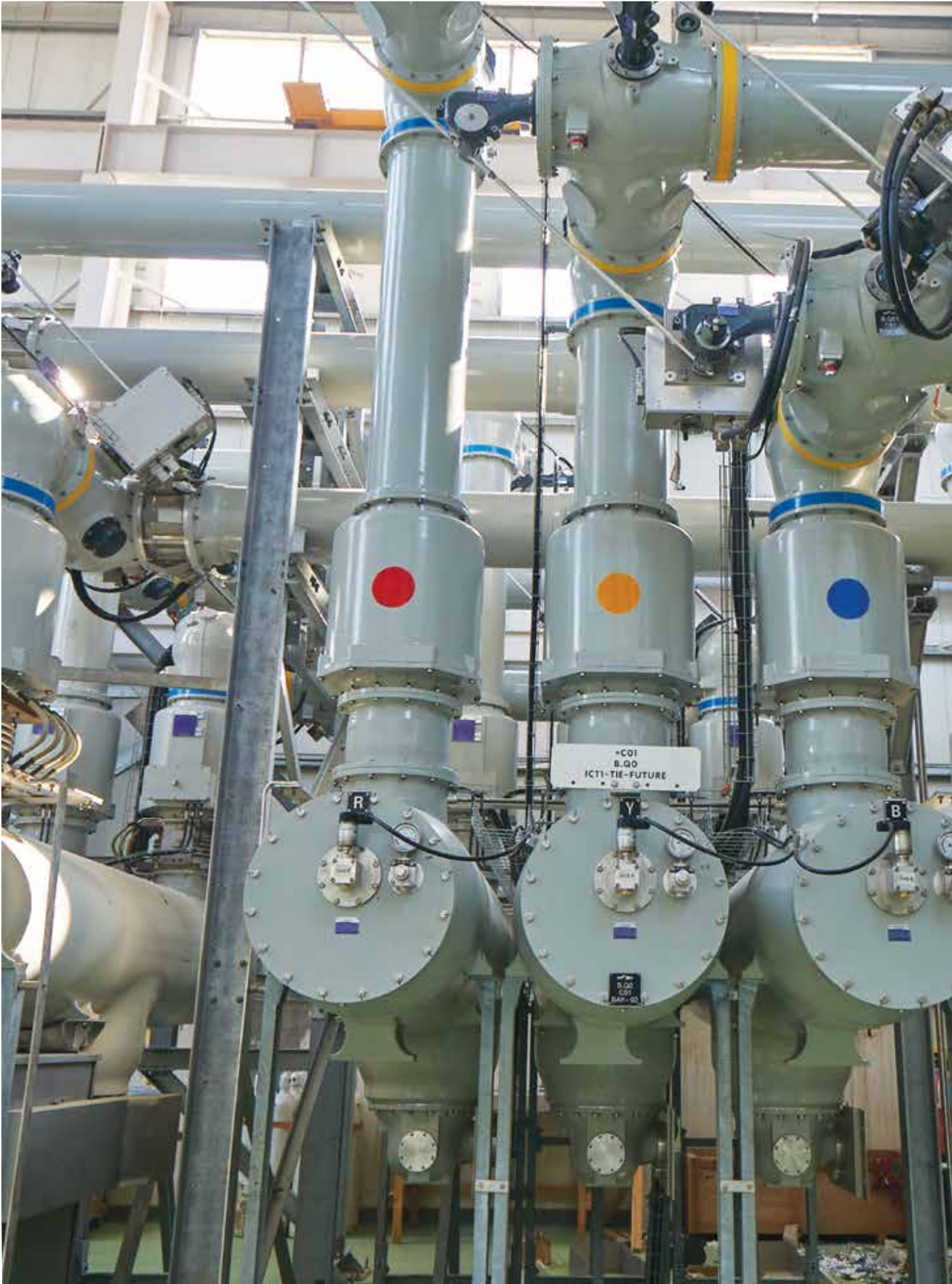
Gas Insulated Substation at 800kV 3000 MW Champa Kurukshetra UHVDC link
