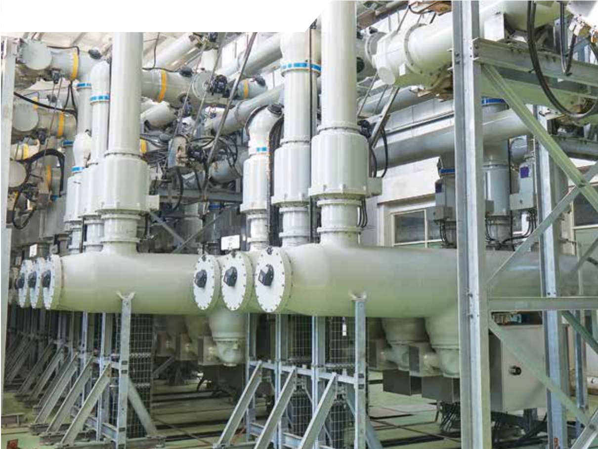
400kV Gas Insulated Switchgear at Kandapalli, Andhra Pradesh
