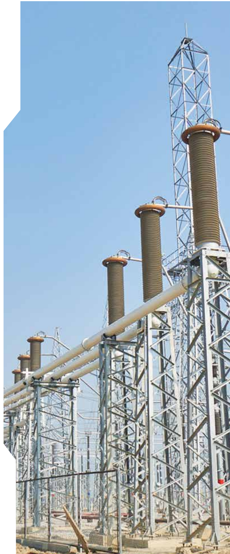
UHVDC Champa Kurukshetra link enabling bulk power transfer of 3000 MW
