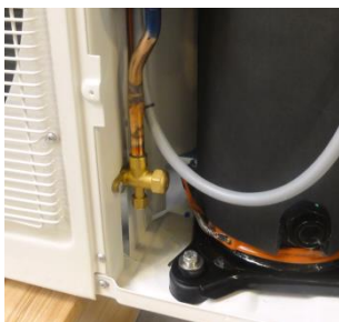
Figure 27: Liquid line service port
