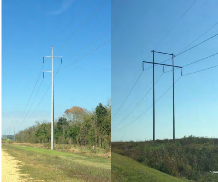
Figure 2-1. Typical Single and Double Steel-Pole Structures
