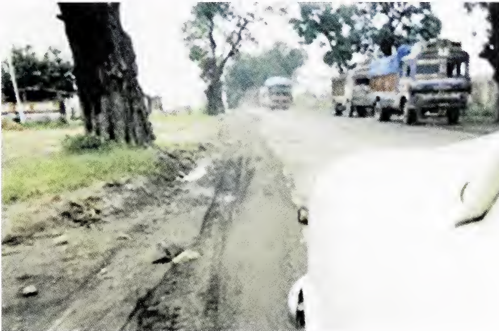
Fig. 5.20 Poorly Maintained Shoulder of Inadequate Width and Strength
