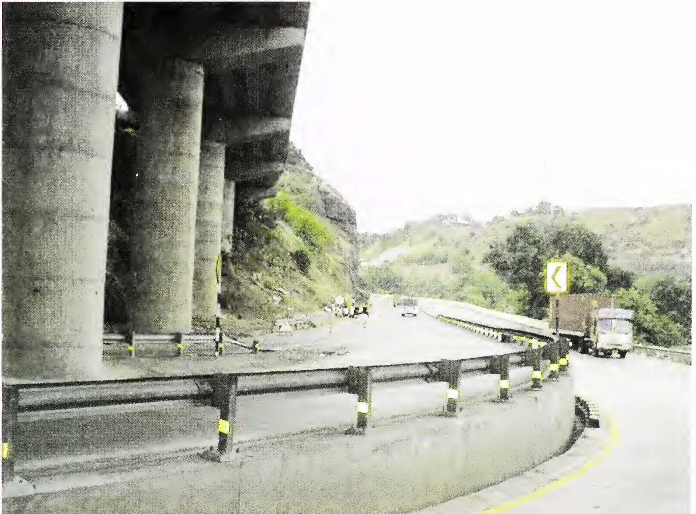
Fig. 5.3 Critical Location Requiring Speed Controls
