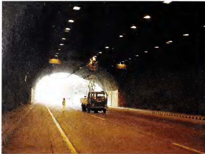
Fig. 5.34 Adequate Lighting should be provided in Tunnels
