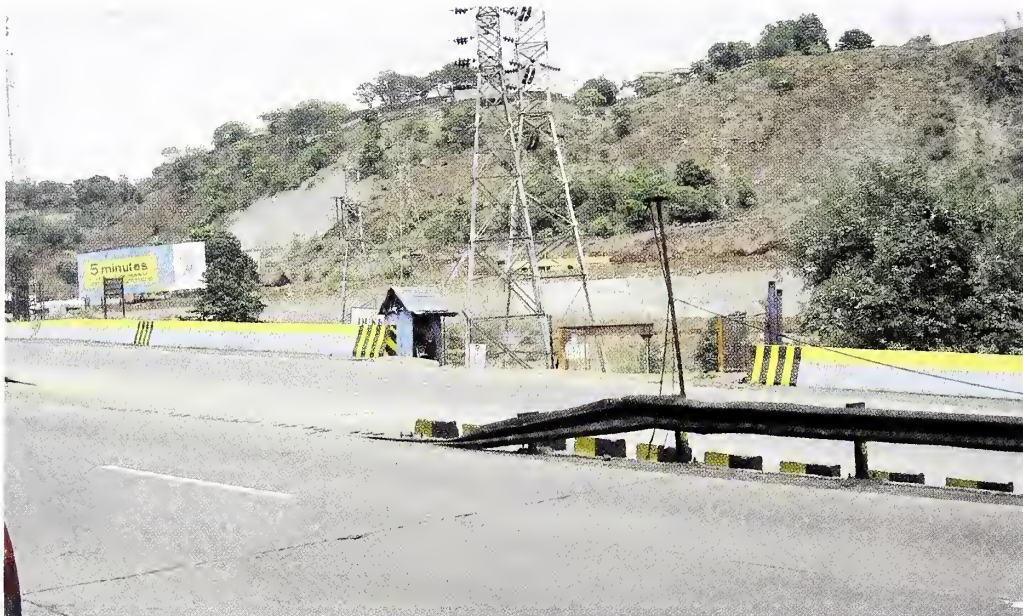
Fig. 5.18 Wrong/Incorrect/Unplanned Opening in the Median Likely to Result in Serious Accidents
