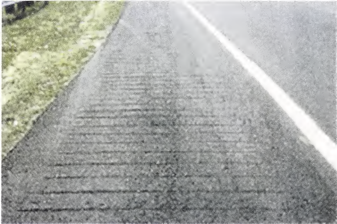
Fig. 5.22 Rumble strips on Shoulder to Alert Drivers who have Strayed from Carriageway before Sharp Curve
