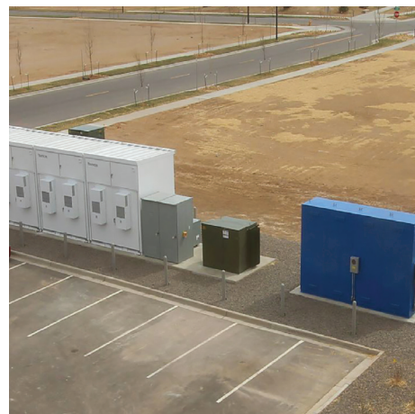
The 1 MW/2MWh battery storage system and associated switchgear.
