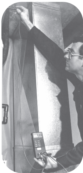
FIGURE 48 TEMPERATURE RISE MEASUREMENT
