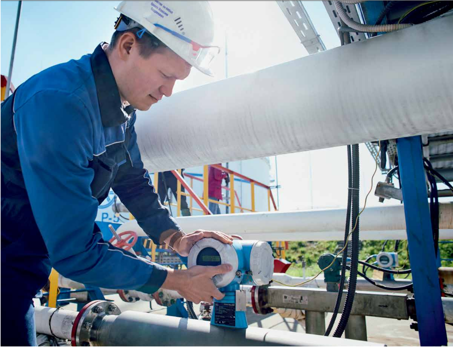
Superior precision during custody transfer: The company relies on Coriolis flow measurement technology for raw materials delivery.
