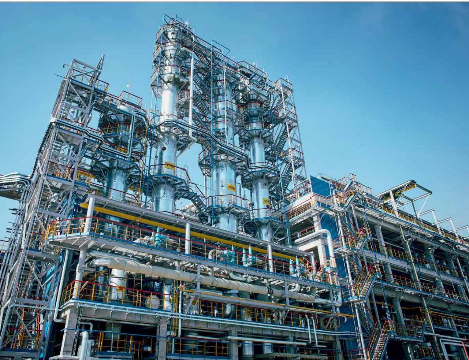
Latest technology and state-of-the-art processes: The ethylene plant will go into operation soon.
