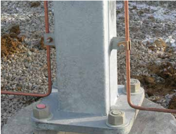
Substation earthing riser
