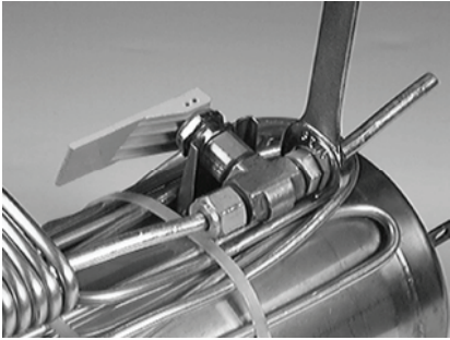
Figure 19: Vent Extension Tube Removal
