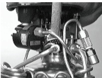
Figure 17: Warming Coil Removal
