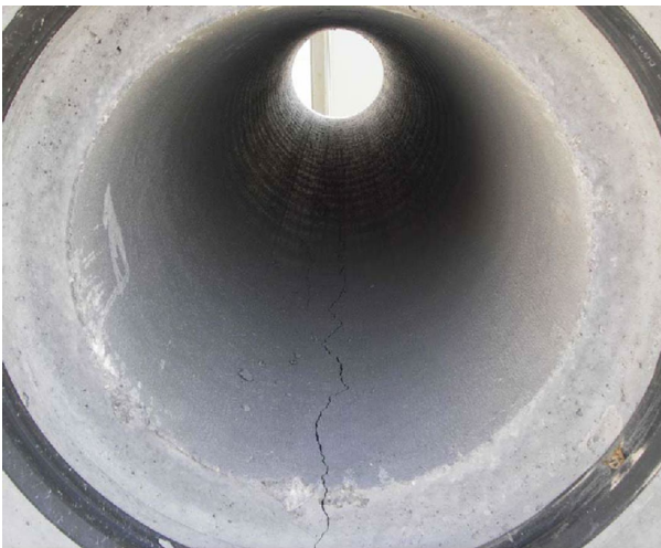
PHOTO NO. 1, Example of Flexural Crack
