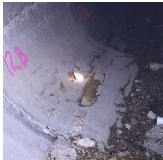
PHOTO NO. 3, Example of Radial Tension Cracks
