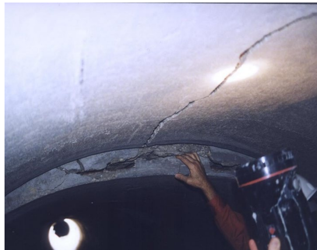
PHOTO NO. 2, Example of Shear Crack
