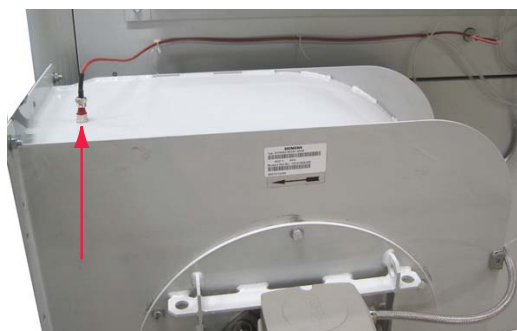
Figure 3.21 PT1000 connection at reactivation fan
