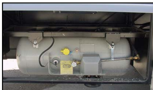
Figure 2-2. Liquid Propane Tank
