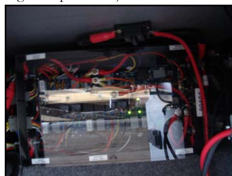
Figure 7-9. Resettable Circuit Breakers
