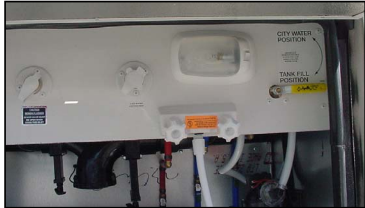
Figure 11-6. City Water Connection
