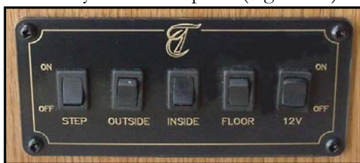
Figure 7-4. Battery Disconnect Panel
