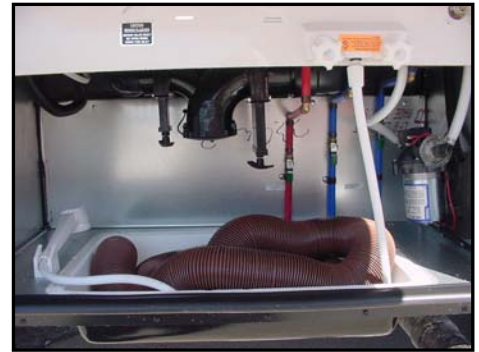
Figure 11-11. Exterior Shower in Outside Sanitation Compartment
