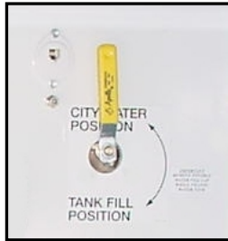
Figure 11-7. Water Fill Valve
