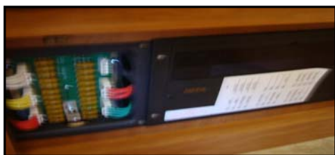
Figure 7-1. Circuit Breaker Box
