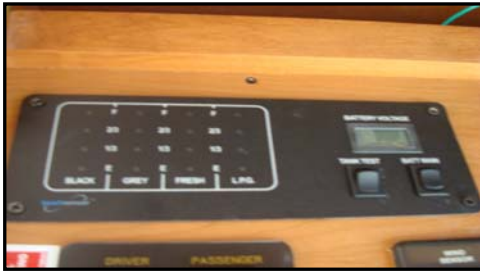
Figure 11-1. Monitor Panel (Water, LP Gas, Battery)
