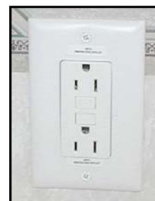
Figure 7-5. Typical AC Receptacle
