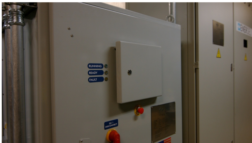
Figure 5-2 Lithium Ion Battery Energy Storage System located at the Black & Veatch Headquarters
