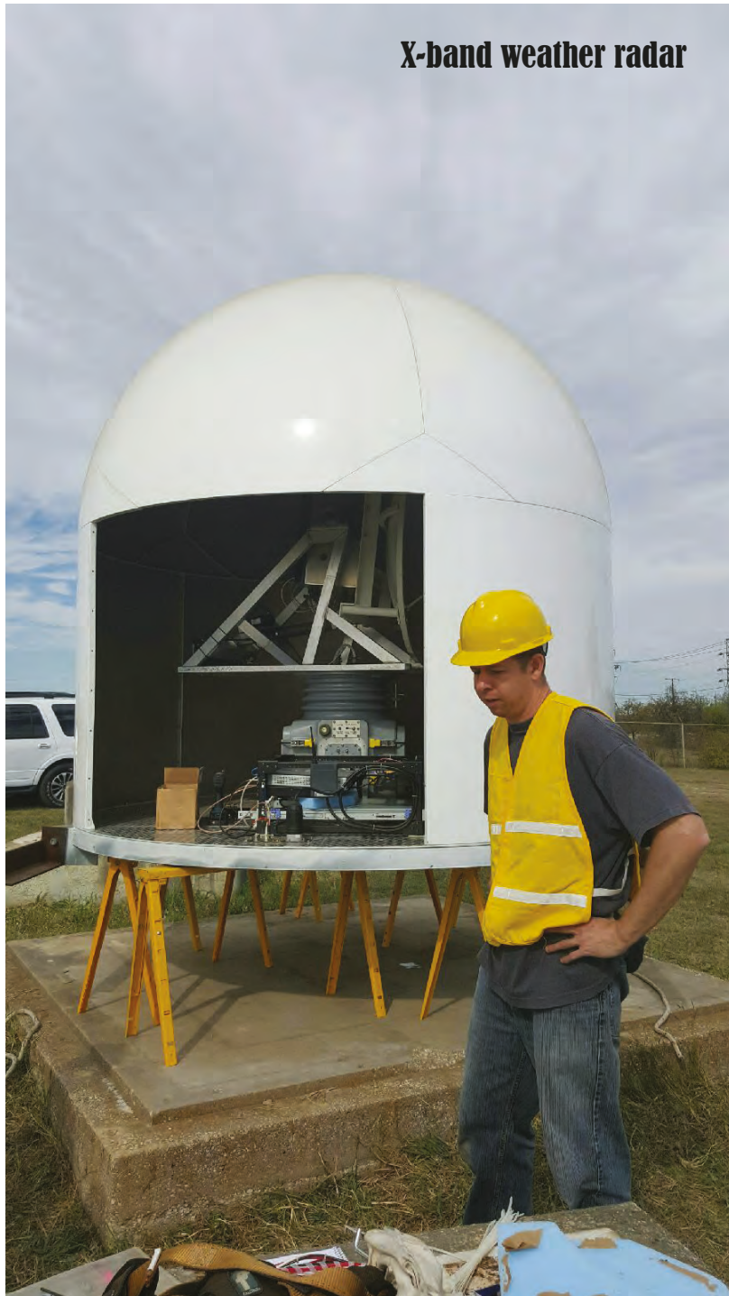
➔ Figure 4: Prepping the CASA radars prior to installation (Image: Apoorva Bajaj, University of Massachusetts)
