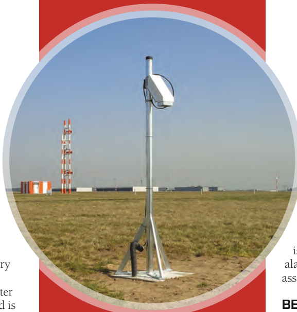
↑ The local installation of at least one field mill per airport is necessary to measure the local electrostatic field
