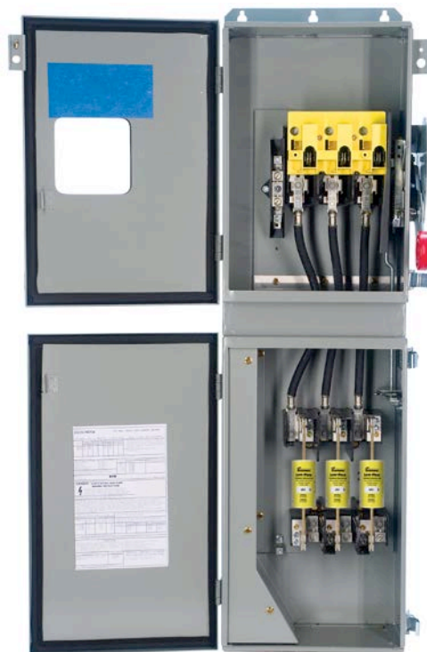
Figure 3. Double-door safety switch
