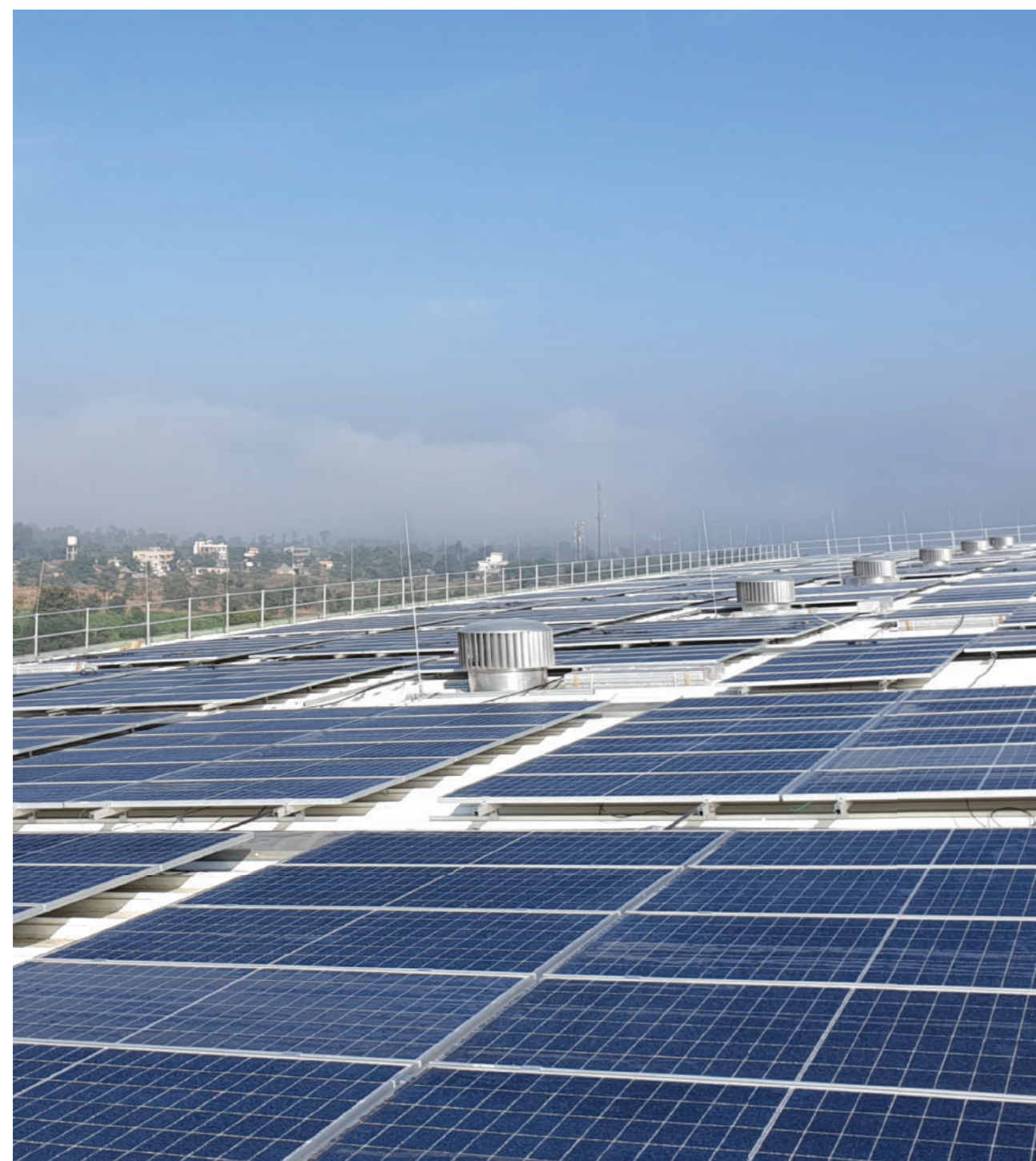
1.5 MW Solar PV installation at Godrej Appliance factory at Shirwal
