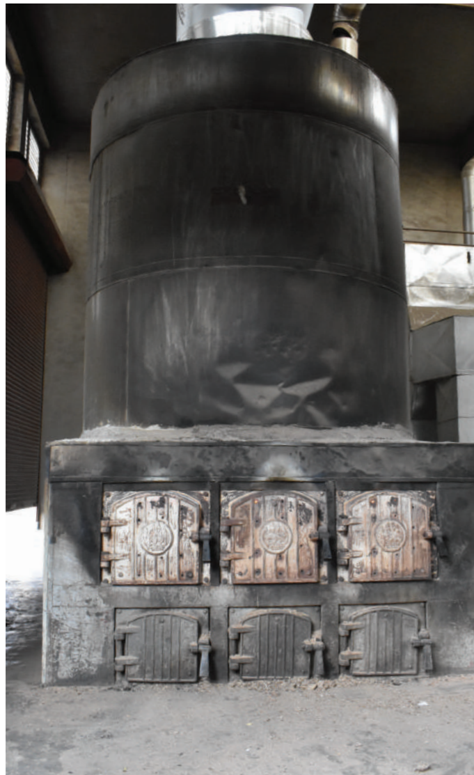
• Thermic Fluid Heater using Biomass as fuel
