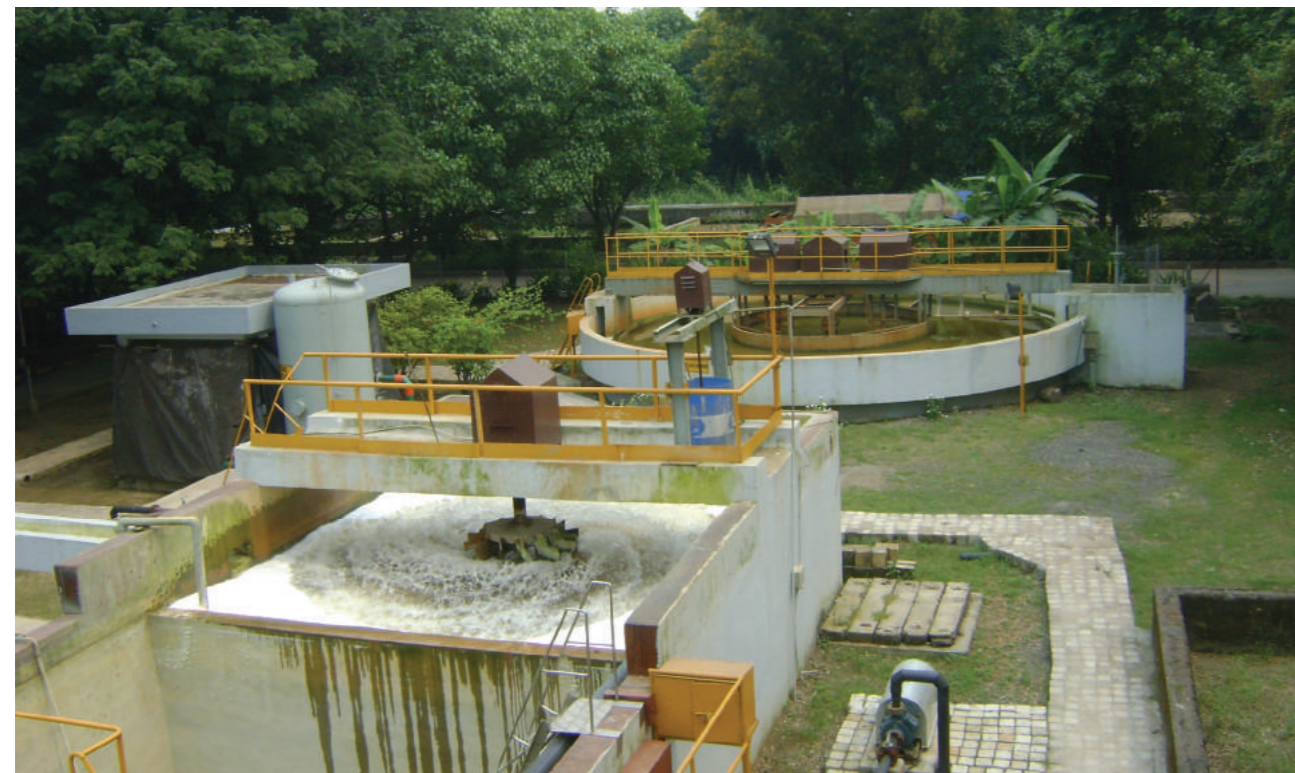
Common Effluent Treatment Plant (CETP) at Vikhroli
